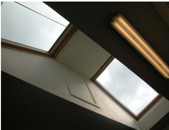
Image 2: Natural and low-energy lighting in changing facilities at Guildtown
