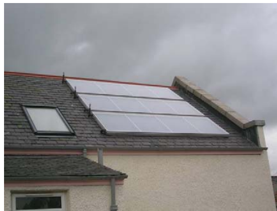
Image 3: Solar collectors to provide hot water on south elevation of extension
