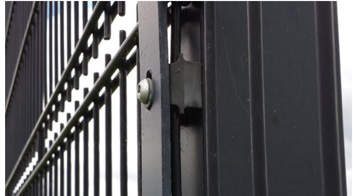
Noise resilient clip retrospectively fitted to fence at Primary School pitch site. Site had been subject of noise complaints from neighbours due to ball being kicked off fence; and after clips fitted; no further complaints have been received.
